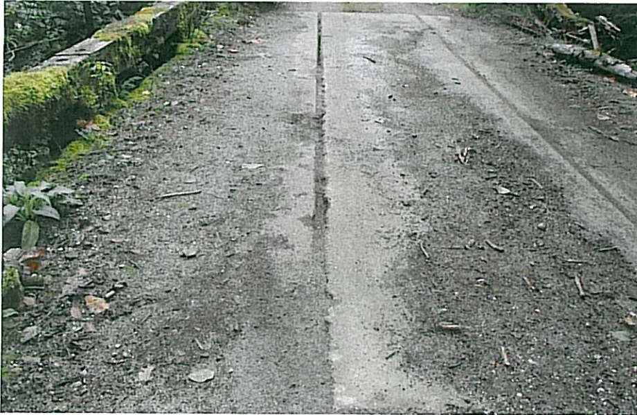
CK-2353 Slab Displaced
